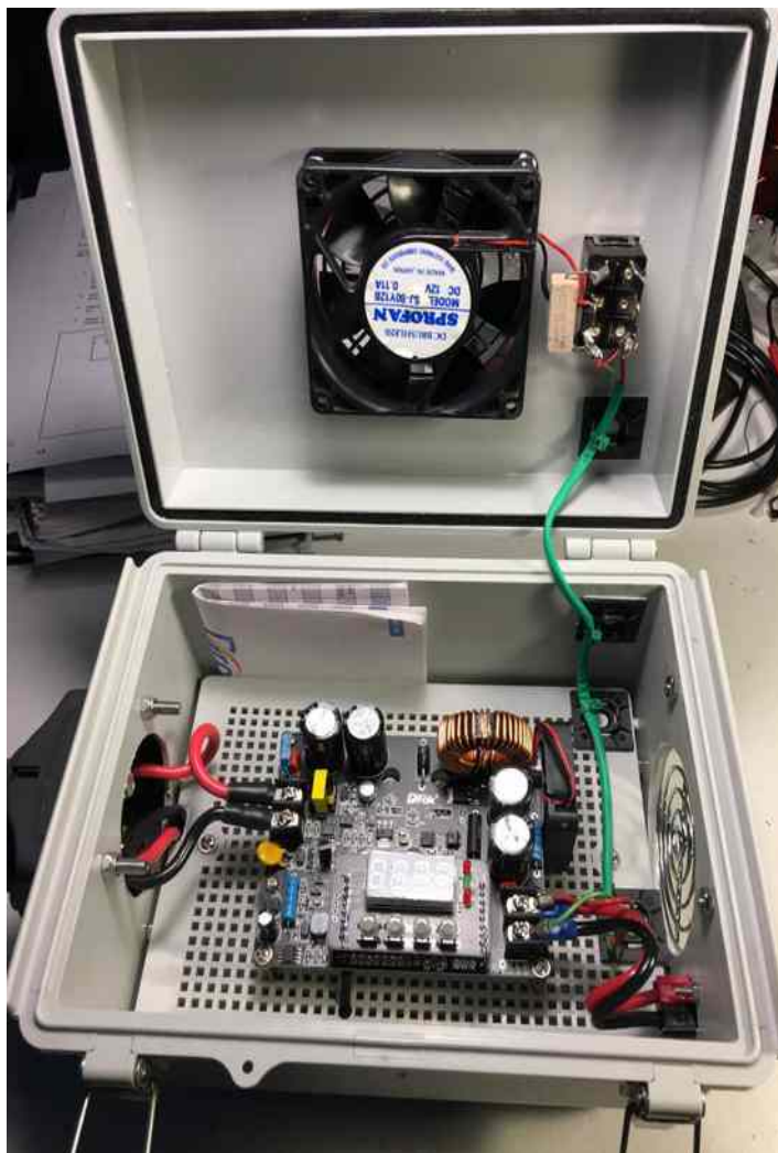
Interior view. Cooling fan blows air down into box.
